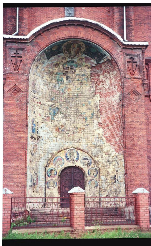
Fig. 5 a, b. Fragment of the Western portal and the general view of the southern exedra. The condition of the majolica. Photo by the author, 1995
